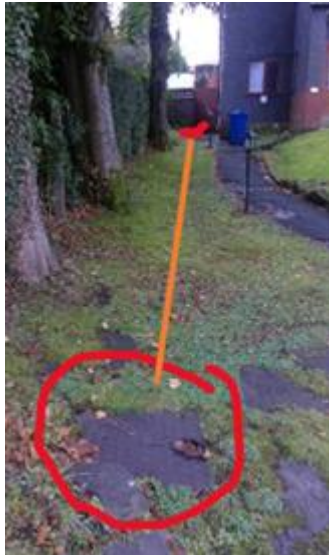
Image 1 – Manhole adjacent to the tree roots leading to the dwelling.
